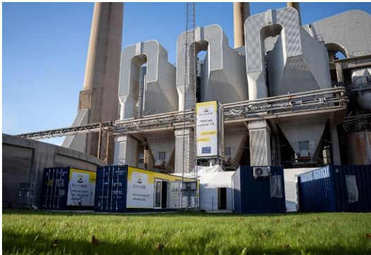
Pilot carbon capture plant at cement plant in Aalborg, Denmark
